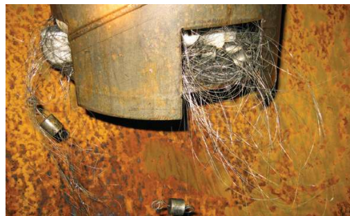
Picture 3.1: Unreliable mechanical level transmitter (servo type)
