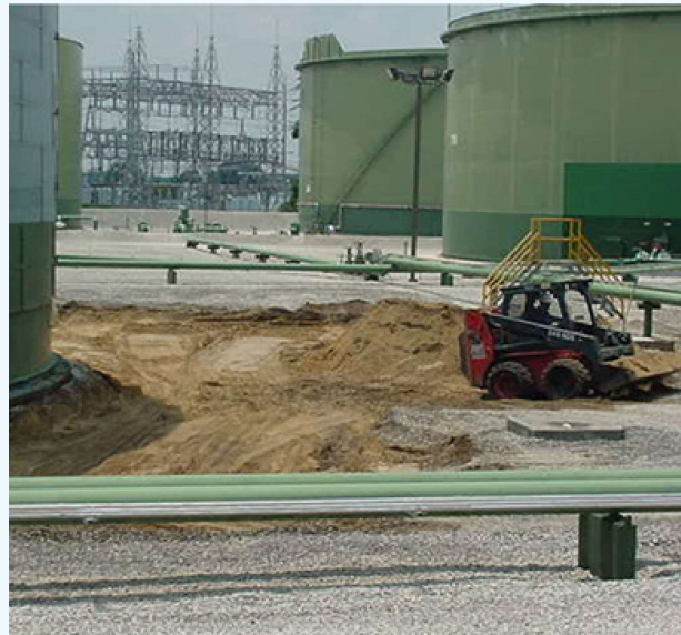
Picture 2.2: Spill clean up
